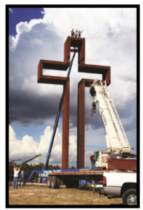
On 7/27/10, the $2,000,000 Corbin steel 17' tall symbolic cross was finally erected on its $100,000 concrete foundation after a two year delay, due to attacks from atheists and other adversaries of the cross. After a difficult $200,000 legal battle, which drained TCKF of their funds, Eagle Bronze of Lander, WY and other area contractors volunteered their time and donated their profits to raise the cross on the mountain for Jesus Christ! Christians around the world watched LIVE, streaming of this historic event.
